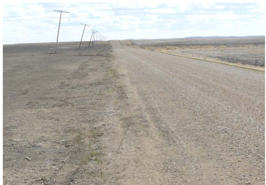
Soil from water going right up to road and power poles starting to lean over due to wet ground and water pushing
